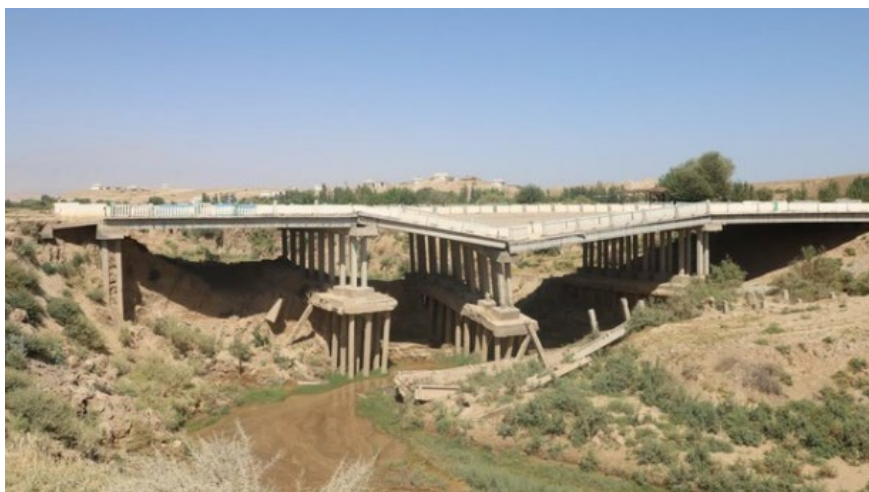
Figure 4 - An example of a collapsed bridge
