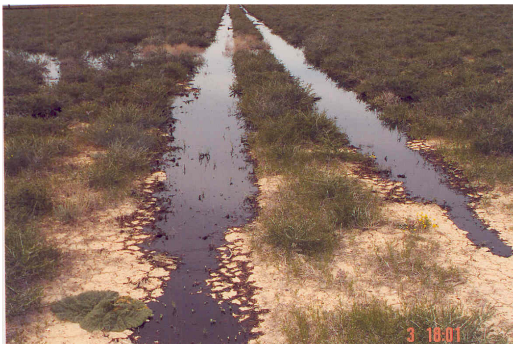
Figure 2 - An oil-contaminated area of a main oil pipeline
