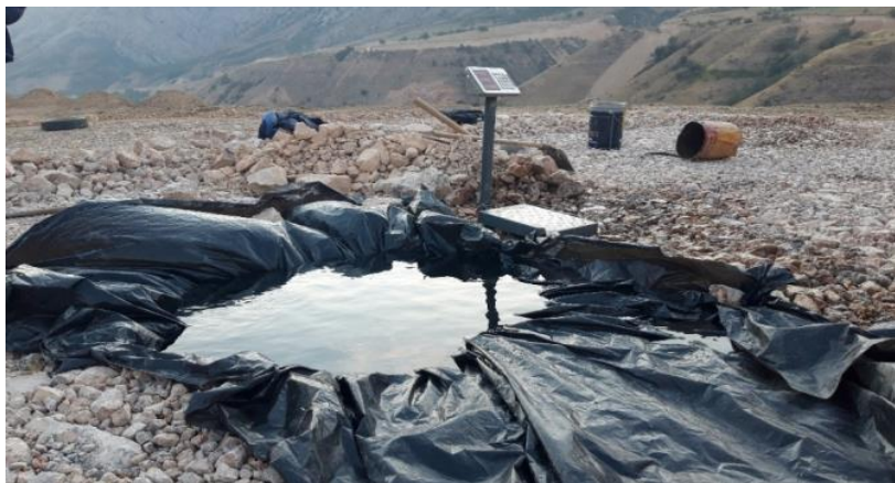
Figure 1 – Determination of density using the “pit-hole” method of the first layer after two passes with a smooth roller with a vibrator turned on
