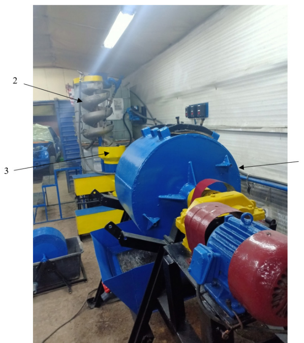
Figure 1 – The aggregate technological installation for processing mineral samples. 1 – autogenous mill; 2 – screw separator; 3 – vibrating centrifugal bowl-type units.
